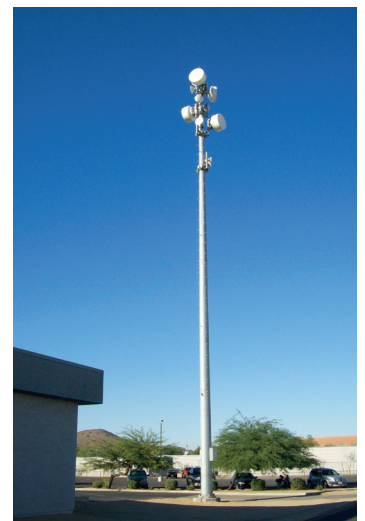
100 foot-tall monopole at the District Administration Center (DAC) connects to the District's other 46 campuses. (Source: NIC)
